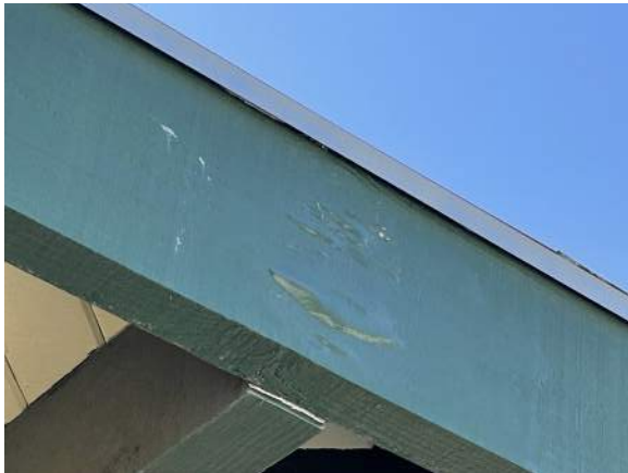
example of bubbling at wood fascia
