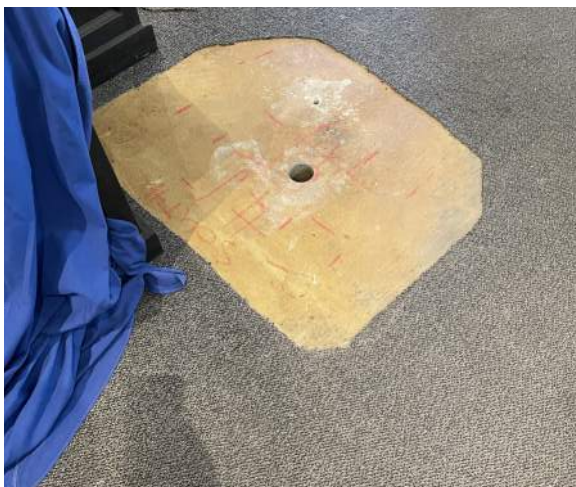
Section of carpet removed at gift shop floor for concrete core sampling
