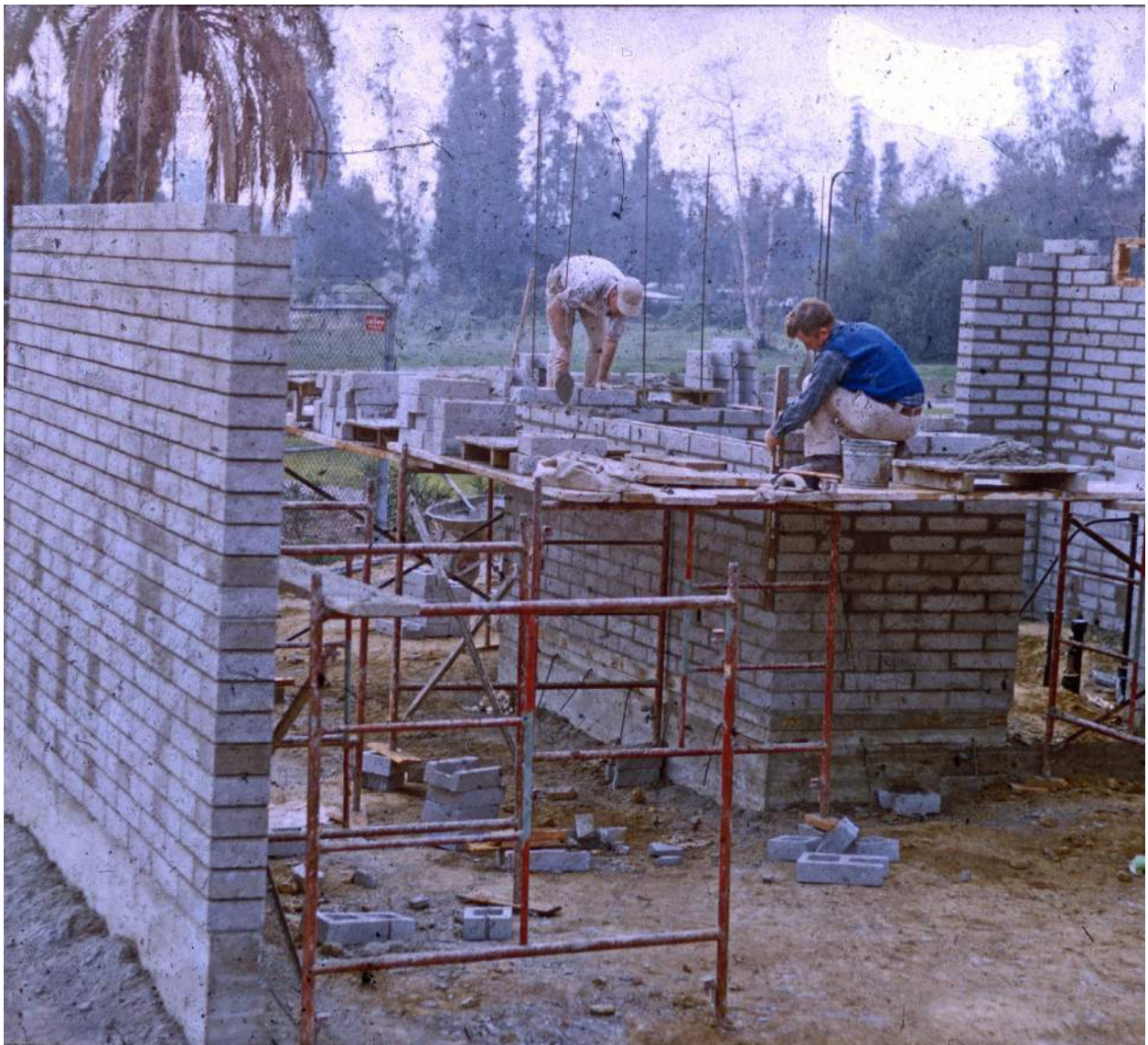
Photo of Gate House in construction. (photo credit: William C. Aplin, 1955 courtesy of Los Angeles County Arboretum Archives)
