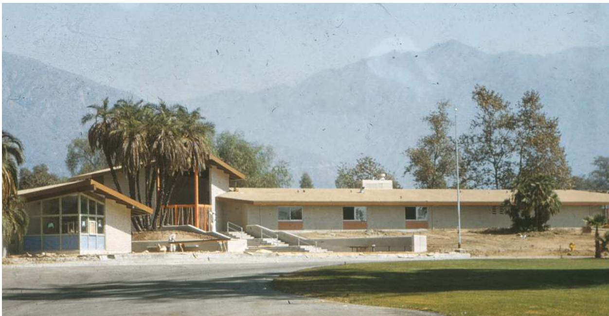
Photo of Gatehouse and Administration Building in construction, view looking north. (photo credit: William C. Aplin, 1956 courtesy of Los Angeles County Arboretum Archives)
