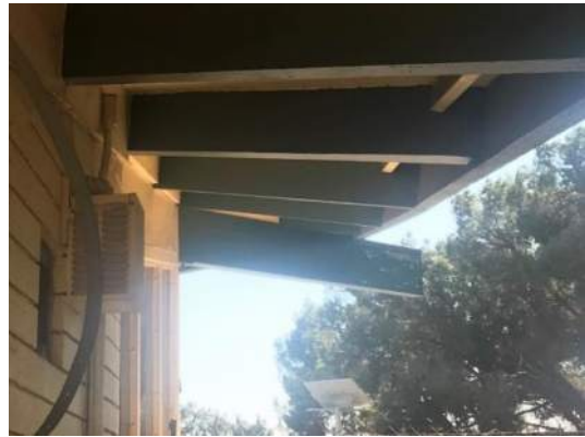
Figure 3 - Roof rafter tail deterioration
